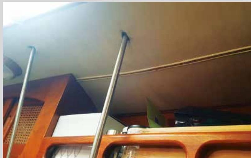
The chainplates, backing plate, and tie rods are accessible under a vinyl headlining
