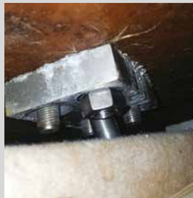
The chainplate below deck consists of a pair of U-bolts, aluminium backing plate, and stainless steel tie rod
